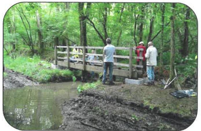
Volunteers helping the Senior Rights of Way Warden replace a bridge in the New Forest National Park
